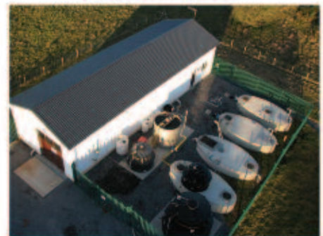
Milltown WTP, Co. Galway
