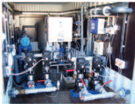
Burishoole Temporary WTP, Co. Mayo
