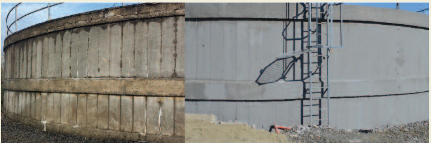
Before and after pics of reservoir refurbishment work completed by InDepth Water Management.
