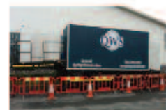
QWS Mobile Pumping Unit
