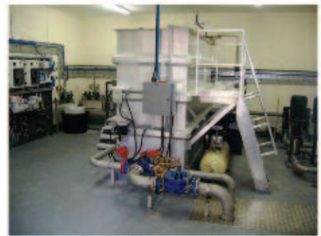
Castlebaldwin WTP, Co. Sligo
