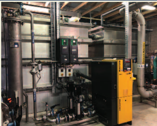
The upgraded DBO water treatment plant at Brackloon/Spaddagh GWS, one of many projects completed under the Rural Water Programme capital investment programme in 2017.
